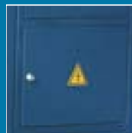
Current outlets for power tools and measuring instruments.
