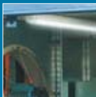
Fluorescent luminaires on either side of the engine.
