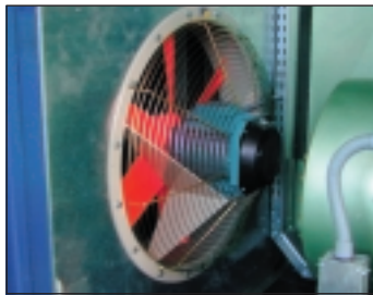
■ Container and auxiliary services for the genset
